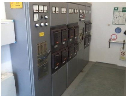
(Trafostation am Weinberg)
